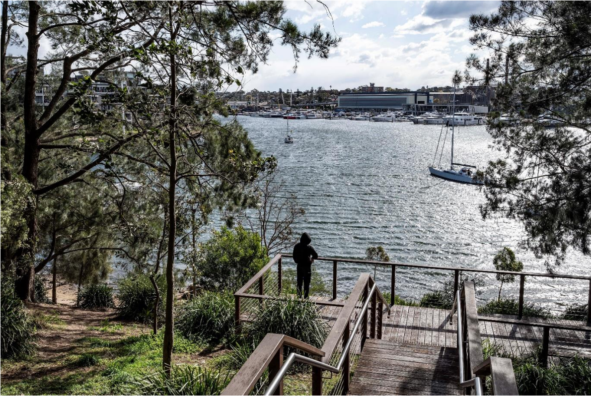
Existing timber deck and stair access to the Glebe foreshore walk be repaired
